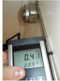
Figure 2: Air flow measurement showing air leaks at the fire extinguishing outlet
